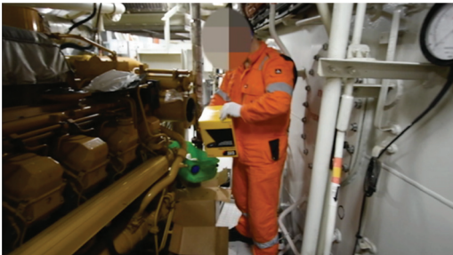
Figure 1. Absence of working surface on the engine. The mechanic needs to place the tools and spares directly on the engine.
