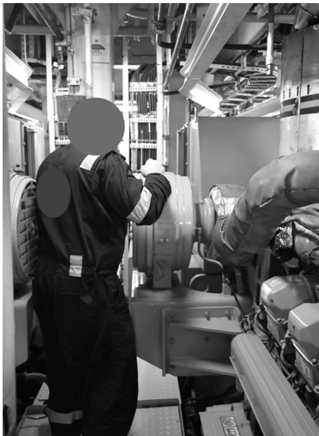
Fig. 4 A crew member shows the narrow passage between two engines
