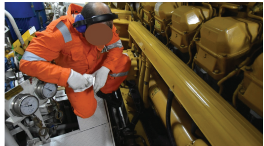
Figure 4. Constrained space around the engine, lack of body support and non-ergonomic body position. The mechanic is resting his elbow on pressure and temperature gauges that are not designed for carrying weight. Both his feet are only halfway resting on the flooring.
