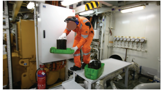
Figure 3. Risk of head injury, trip, and fall, as well as oil spill. While carrying used oil filters in a receptacle full of oil, the mechanic needs to climb down stair steps while bending his back and knees to avoid hitting a beam with his head.
