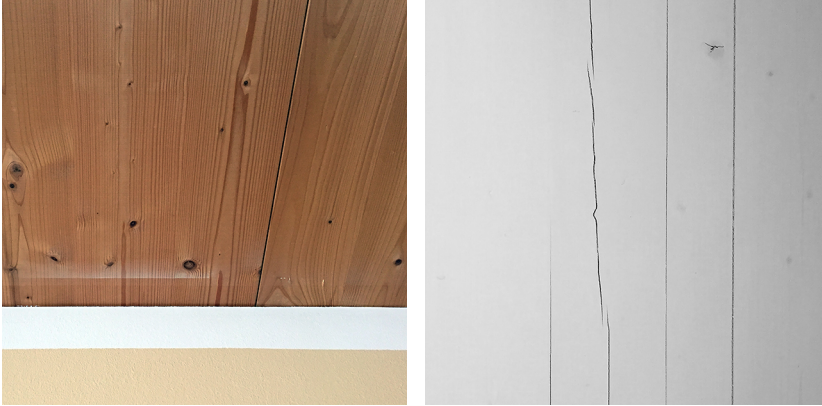
Figure 2.9 a) Gaps between CLT slab elements at Mühlweg (A), and b) cracks in the CLT walls at Skadbergbakken.
