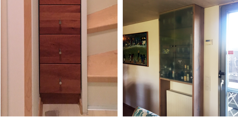
Figure 2.12 a) Tailor-made seizing of gaps and spaces around a stair at Mühlweg (B), and b) around a radiator at Lobaugasse.
