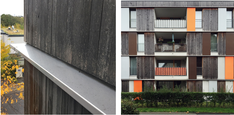
Figure 2.5 Fire safety façade detail, interrupting air flow behind the façade and at the same time becoming a design element in line with shutter guiding rails at Mühlweg (A).
