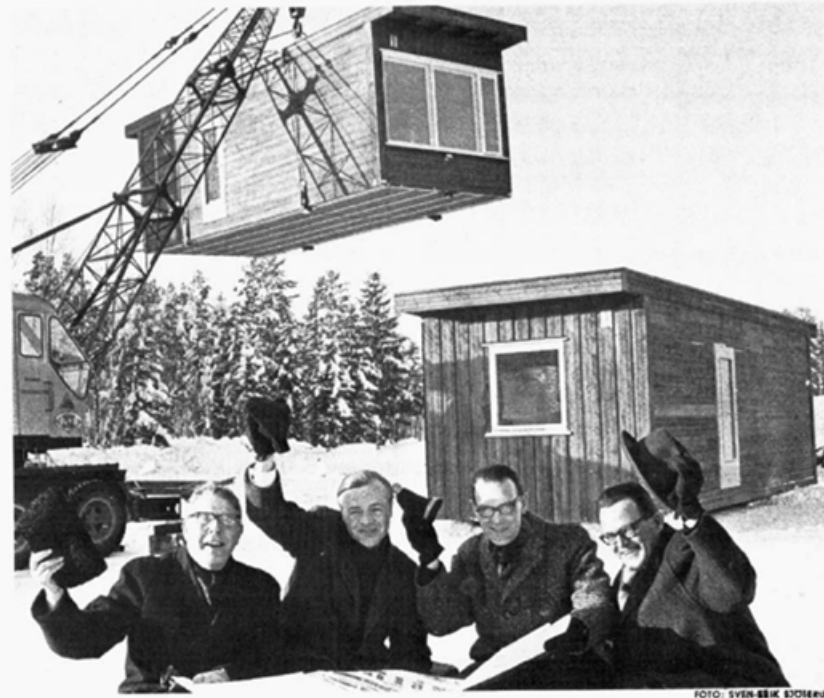
Fig. 8. Moelven section house export to Sweden was very successful. A newspaper headline claiming that the "Norwegian 'people's-villa' is a price-bomb in Stockholm." Newspaper clipping, 1966.
