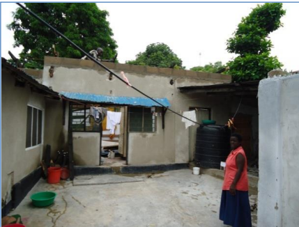
Figure 3.41: Renovation of one of the rooms for rent at Mr. Lusuva's house.
