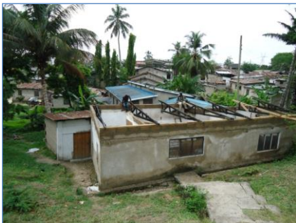
Figure 3.42: The renovation in progress. Mrs. Lusuva's house as seen when approached from outside.
