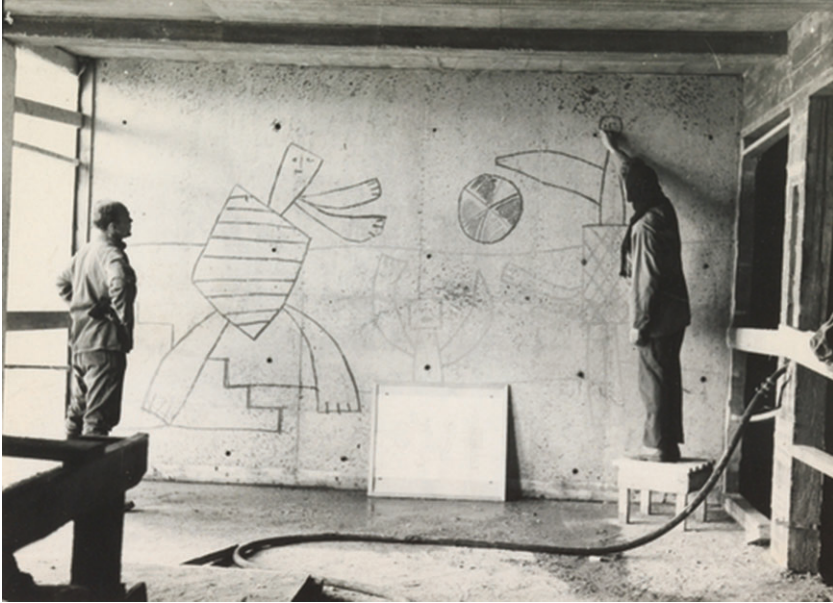
Figure 28. Artwork by Picasso is drawn up on the wall before it will be sandblasted by Carl Nesjar, left. On a landing in the High-rise.
