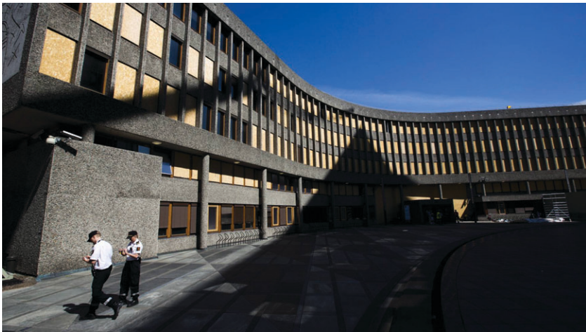
Figure 5. The Y block in 2012, with temporary window covers. Seen from Johan Nygaardsvolds plass.
