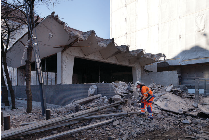
Figure 45. The damaged canteen annex. The draped High-rise in the background.
