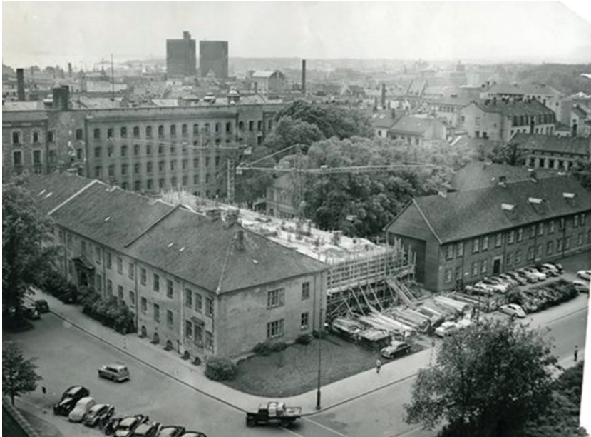
Figure 34. Empirekvartalet with Rikshospitalet and Militærhospitalet. The High-rise is under construction between the buildings. 1956.
