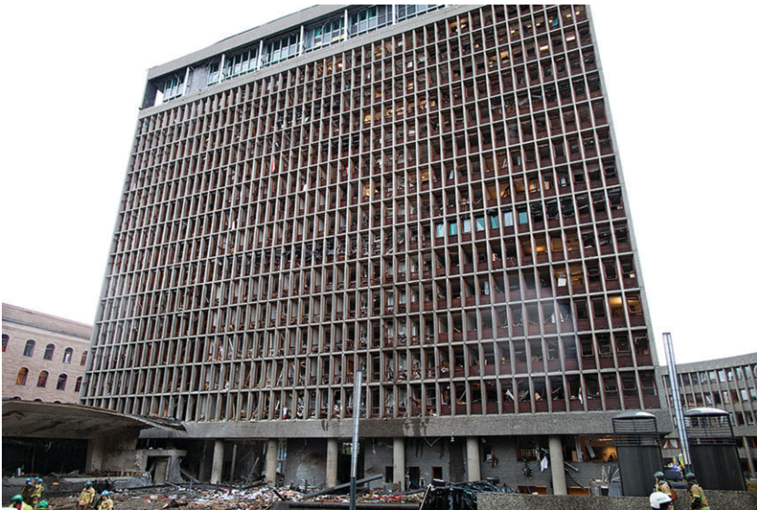
Figure 2. The High-rise after the explosion, seen from Einar Gerhardsens plass.
