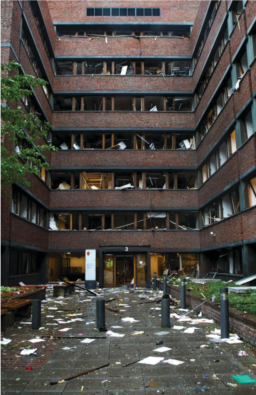
Figure 4. The S block after the explosion, seen from Einar Gerhardsens plass.
