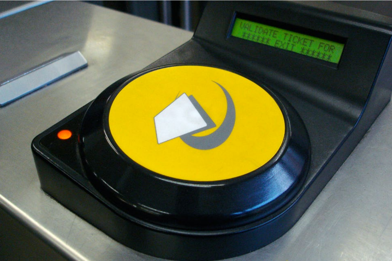
Figure 27: An RFID reader installed at turnstiles on London's Underground system, UK. The image of a card being visually 'swiped' across the bright yellow background offers instruction for how to validate an RFID ticket, while the small, green LCD screen behind provides otherwise invisible information as to the validity and value of each ticket as it is swiped.
