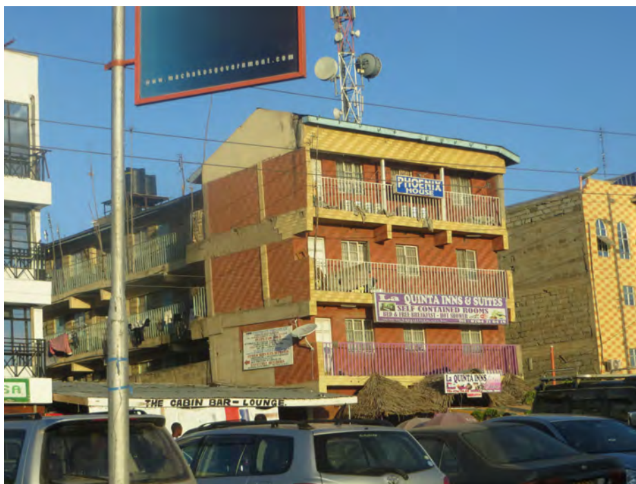
Plate 5.28: The reconstructed façades of partially demolished buildings. Beams are cut and their edges left exposed. Finishes on the fronts of the building differ from those on the side. Partially demolished floor slabs are converted into balconies and extra storage space. (Source: Author)
