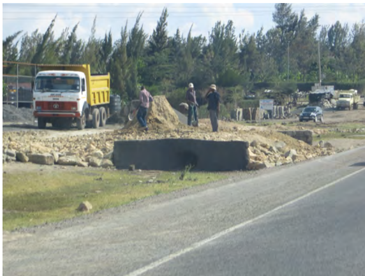
Plate 5.51: Local artisans construct a culvert and access from/into the highway at Utawala. Residents and businesses have been left to connect their own premises to the highway. (Source: Author)
