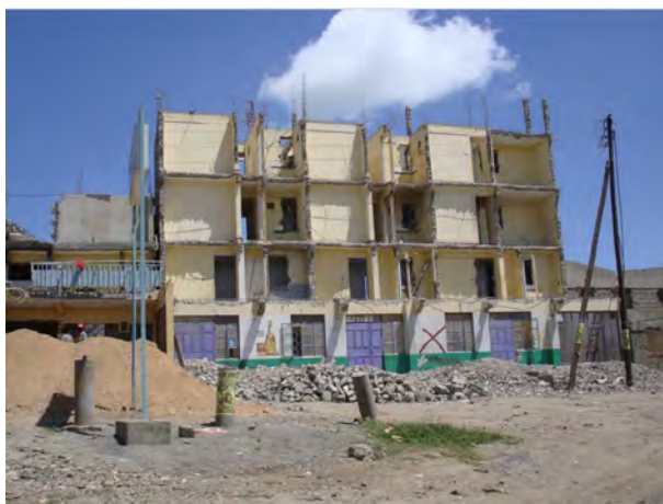
Plate 1.0: A commercial building partially encroaching the road reserve at Mlolongo along the Mombasa Highway in the process of being demolished by its owners on 6 th November, 2006 to make way for highway expansion. (Source: Jamii Forums (accessed on 4 th March, 2015)).
