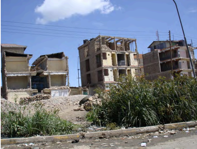
Plate 5.21: A picture showing the partial demolition of roadside buildings at Mlolongo on 2 nd November, 2006. (Source: EGM)
