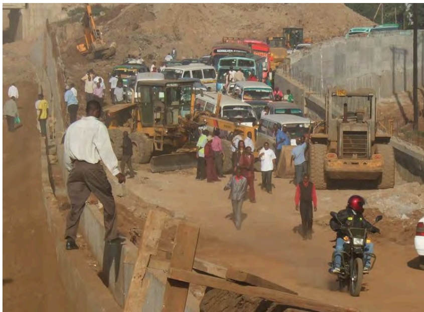
Plate 5.5 The everyday chaos and confusion of pedestrian and vehicular circulation at the Thika Highway during the construction period on 10 th April 2011 (Source: Liz Muthoni and Thika Road Blog).
