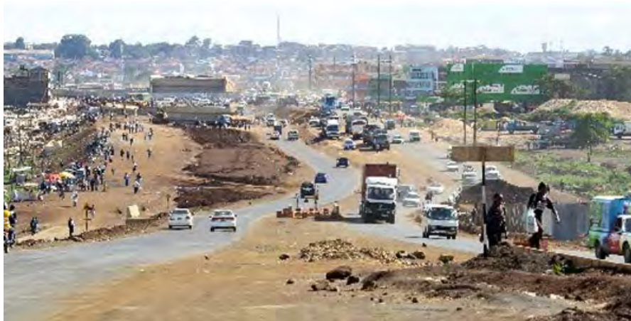
Plate 5.4 Pictures of Thika Highway at Githurai during the construction period on 10 th April 2011 showing the ensuing disruption, confusion and conflicts among traffic modes. (Source: Liz Muthoni and Thika Road Blog).
