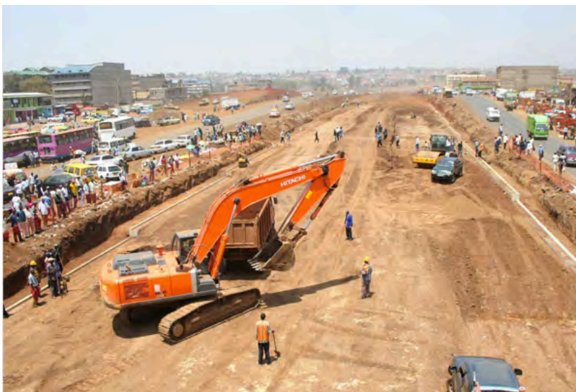
Plate 1.3: Road construction going on at Thika Highway on 6 th December, 2008. Diversions were prepared to cater for vehicular movement but other modes of transport were ignored. (Source: http://www.jamiiforums.com/kenyan-news/231016-the-thika-super-highway-mega-project-21.html (accessed on 9th March, 2015))
