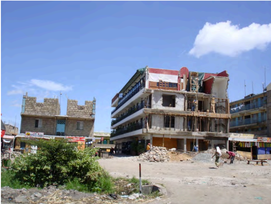
Plate 5.27: Reconstruction of the façade of a partially demolished building in Mlolongo on 12 th December, 2006. (Source: EGM)
