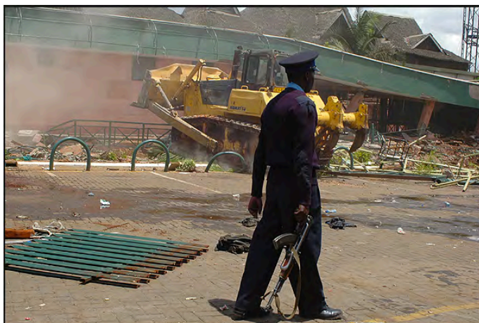
Plate 1.2: An armed policeman watches over a bulldozer and its operator during the forceful demolition of Visions Restaurant on Thika Road at Ruaraka above on 1 st November, 2008 to make way for the transformation of the highway. (Source: Capital FM News)
