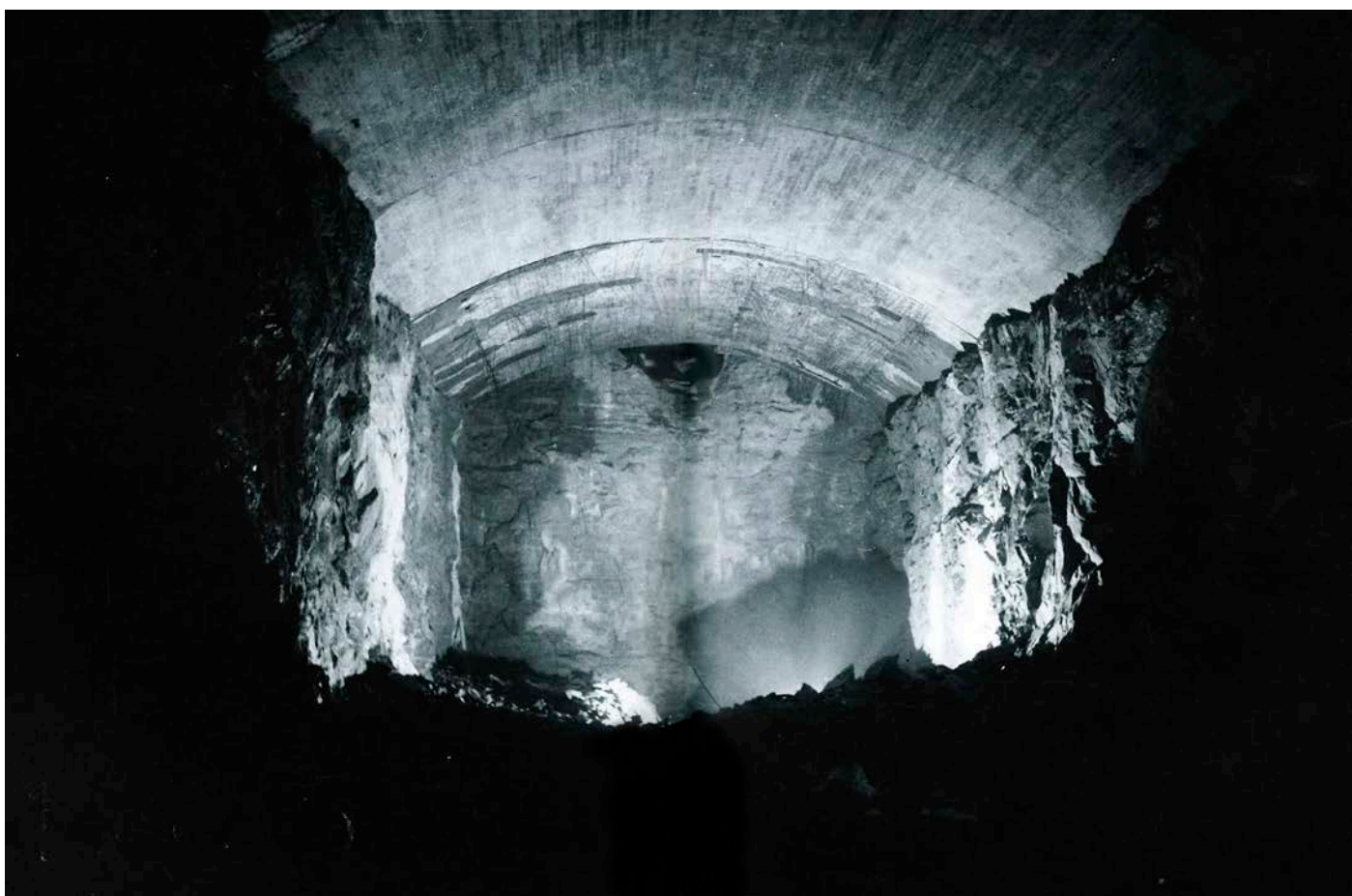
During construction of Lysebotn 1 water power facility. Showing the concrete vault. This is my inspiration for the task.
