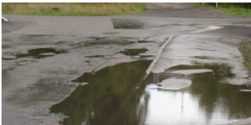
Flooding of infrastructural area
