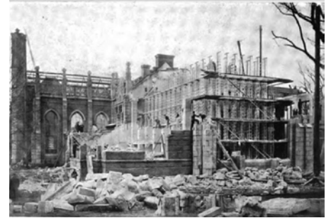
Gore Hall, Harvard University, 1913. 10-Tiered Stack structure is independent of the exterior walls.
