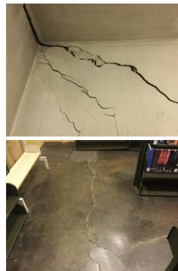
Paint peeling from rising damp the lower walls; large cracks developing in the basements.
