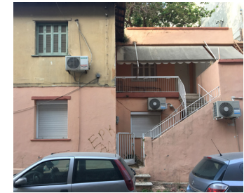
2 Example of abandoned residential building in a neighborhood where refugees rent private apartments.
