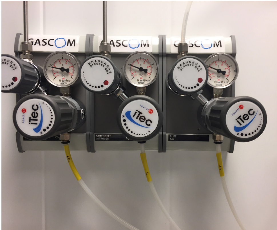
Controls for gas intake
