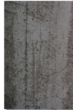
pre-cast concrete column
