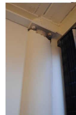
load bearing steel beam covered with fire isolation
