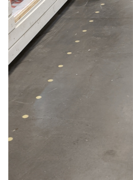
The teachers and students prefer concrete floors in the workshop: durable and easy to clean
