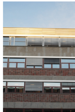
The facade consist of horizontal bands made of: concrete, steel, terracotta tiles and steel window frames. Similar to the facade of Brenneriveien 11.
