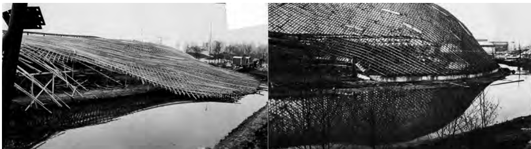
Figure 115 Frei Otto, Carlfried Mutschler and Partners, 1975, Multihalle Mannheim . The laths being deformed to the desired shape.
