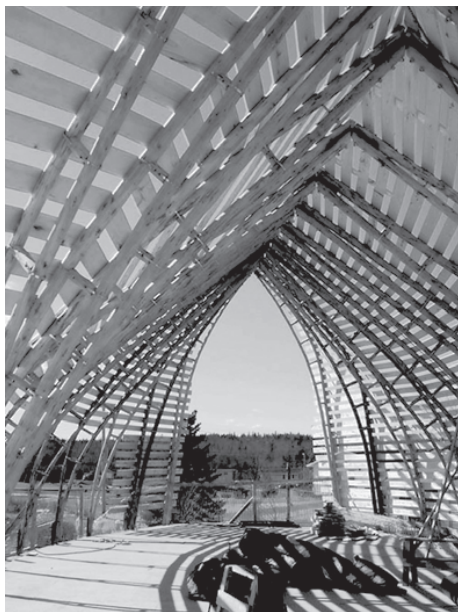
Pictou Landing Health Centre in Nova Scotia, architects Brian Lilley, Richard Kroeker, Peter Henry. Photograph R. Kroeker, from KROEKER, R. 2013. Lernen vor der Architektur der indigenen Volke Amerikas. Learning from Native American Architecture. Detail , 5.
