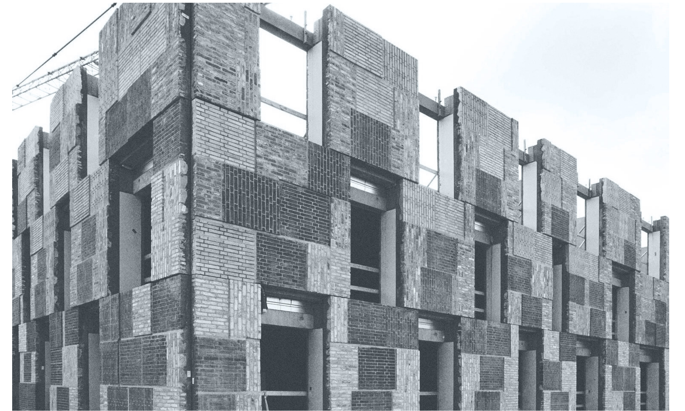
08. Residential project in Copenhagen, Denmark. Brick from local demolition was cut into panels and reinstalled to form the facade.
