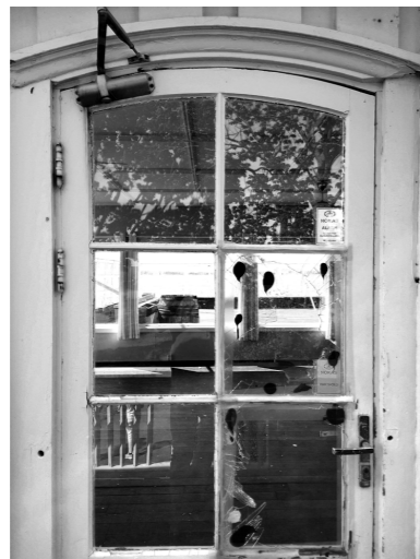
Worn down materials, broken windows, shabby look
