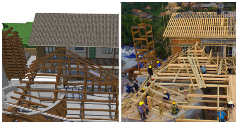
Figure 5.47: The image on the left shows the architect's digital drawing provided to the craftsmen, and the photo on the right shows the actual construction. The craftsmen would revise or propose a more stable and efficient structural system if their experience told them this was necessary. (Source: Author)
