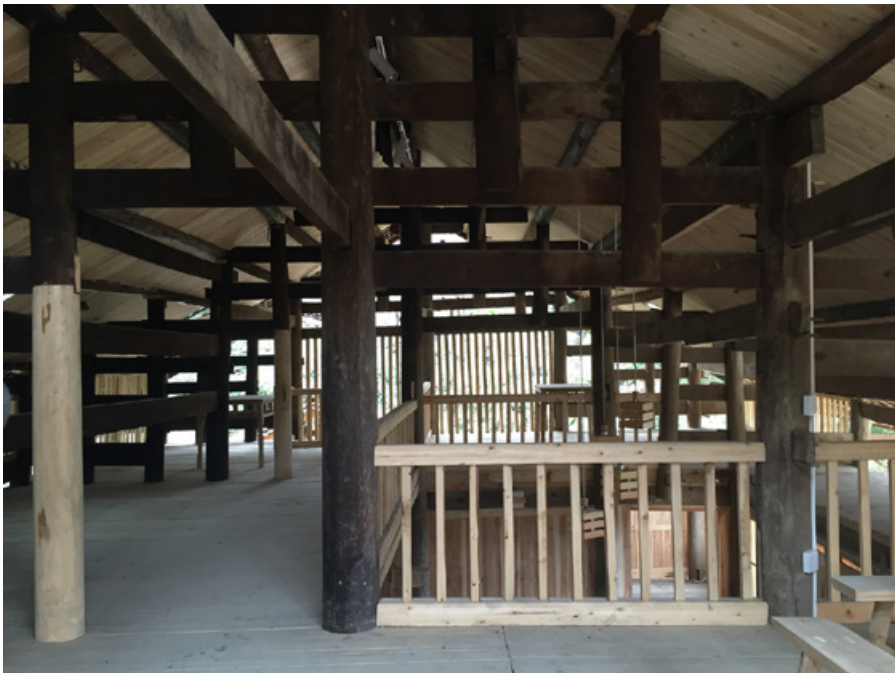
Figure 5.70: The unpainted wooden structures were added to resolve the structural instability caused by creating a corridor in the upper level of the building to enable people to pass through. The photo was taken on November 18, 2016. (Source: Author)
