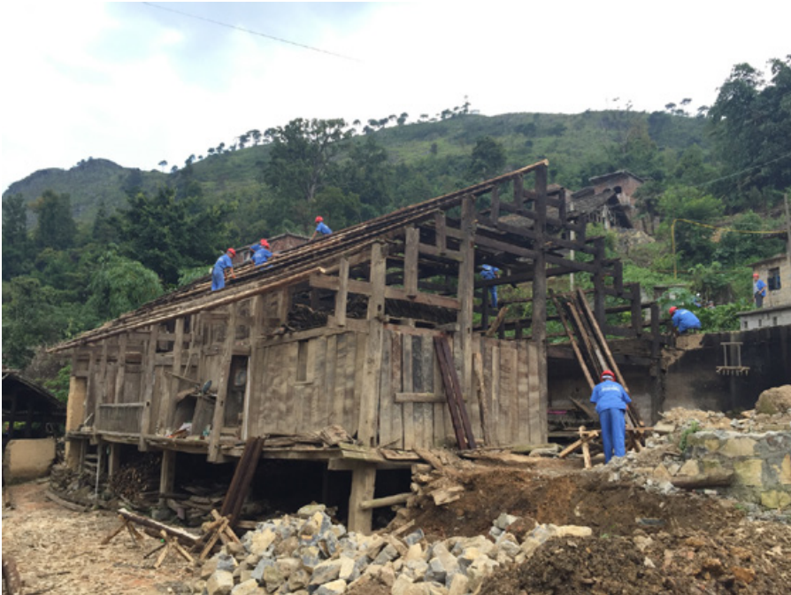
Figure 5.34: The construction workers replaced the decayed rafters and purlins with new ones. The photo was taken on August 29, 2016. (Source: Author)
