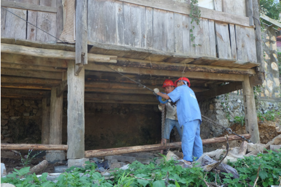
Figure 5.33: Two workers using a simple but effective method to straighten the inclined structures of a stilt dwelling. The photo was taken on September 2, 2016. (Source: Author)
