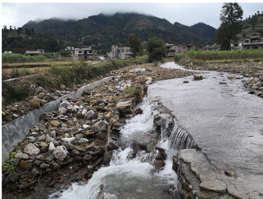
Figure 5.86: The construction of the parking lot severely damaged the irrigation channel. The channel had still not been repaired in late 2019. The photo was taken on November 9, 2019. (Source: Author)
