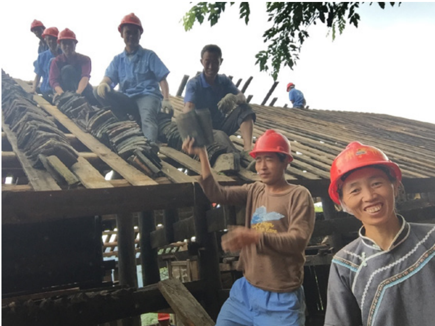
Figure 5.36: Local villagers contributed their labor to their own community. The photo was taken on September 5, 2016. (Source: Author)
