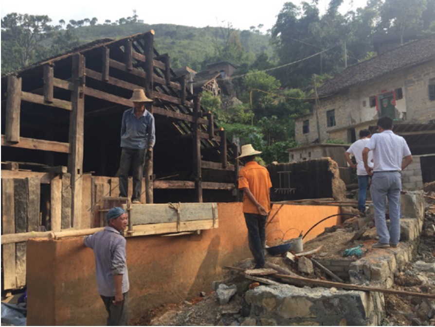
Figure 5.35: Traditional rammed earth wall techniques represented experimental operations undertaken by craftsmen who made effective use of local materials, available tools, and microclimate. The photo was taken on October 17, 2016. (Source: Author)
