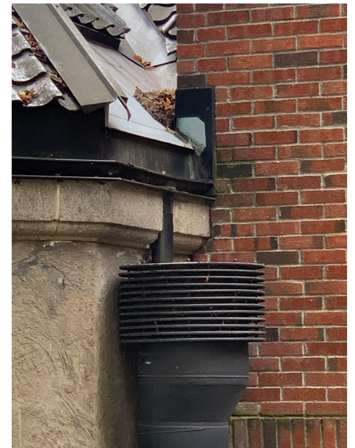
The gutter slices the granite stone to bring the water off the roof.
