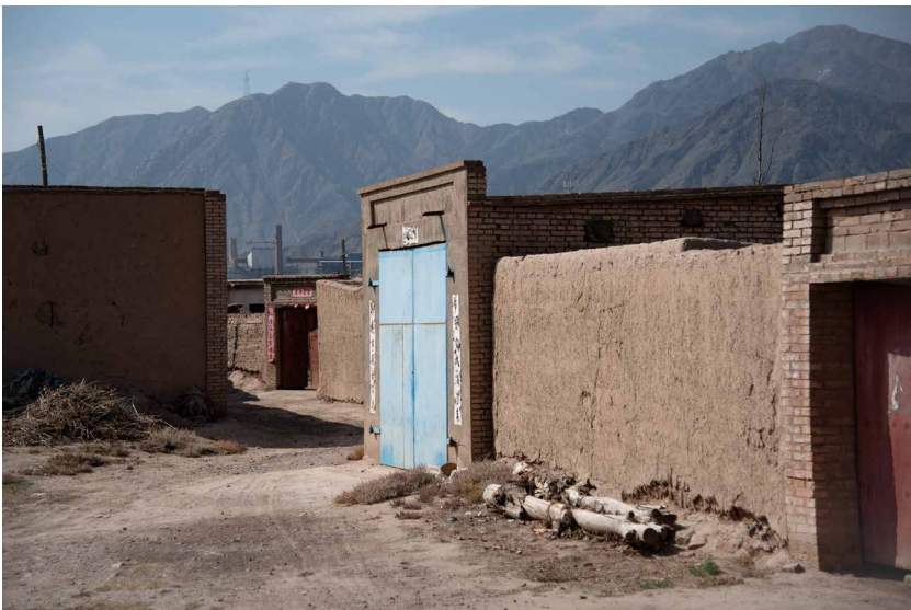
Fig. 4.13: Vacant and decaying homes in mostly empty villages. Rural hollowing in Hexi Pu, Jin-chang, October 2019.
