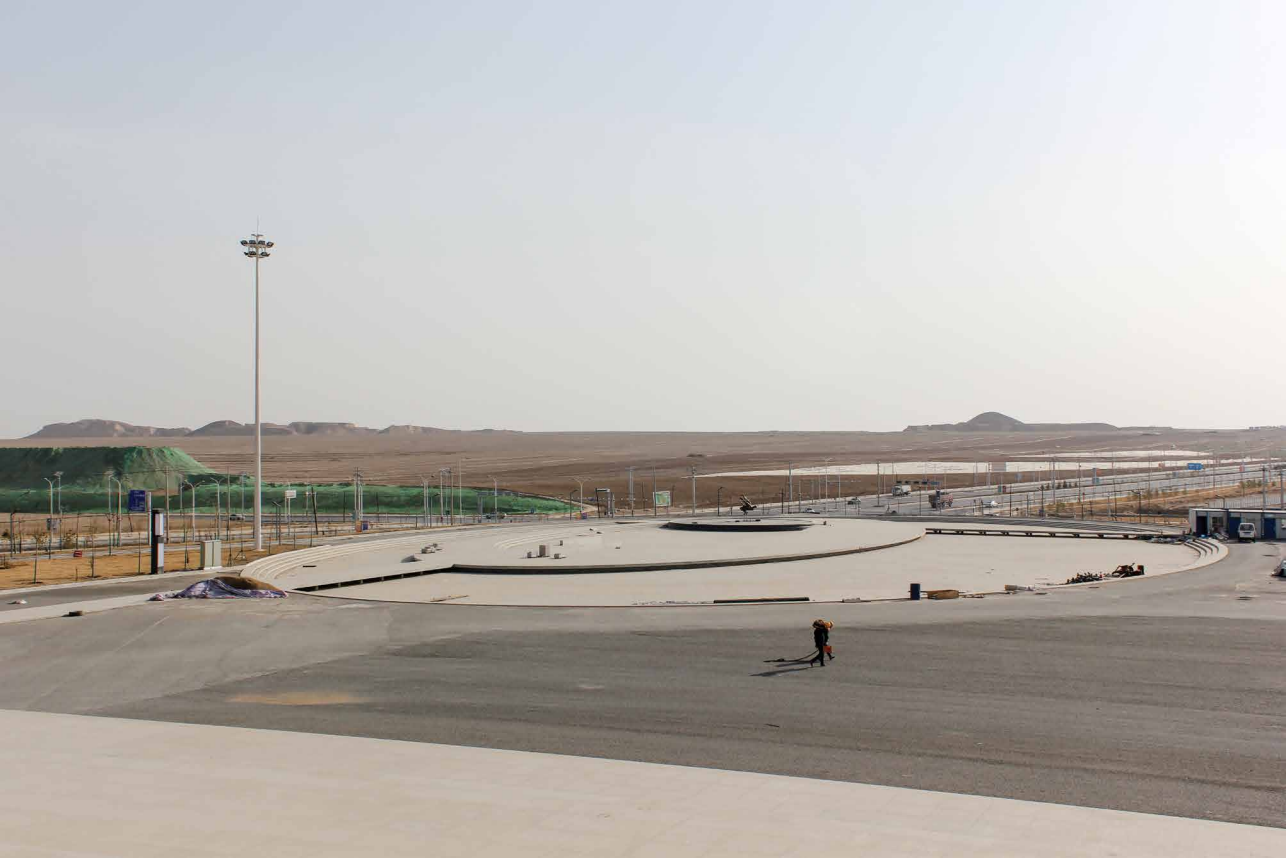
Fig. 5.4: View over the construction site of a plaza with a vast, open plain in the background created by flattening hills and removing villages and farmlands; March 2019.
