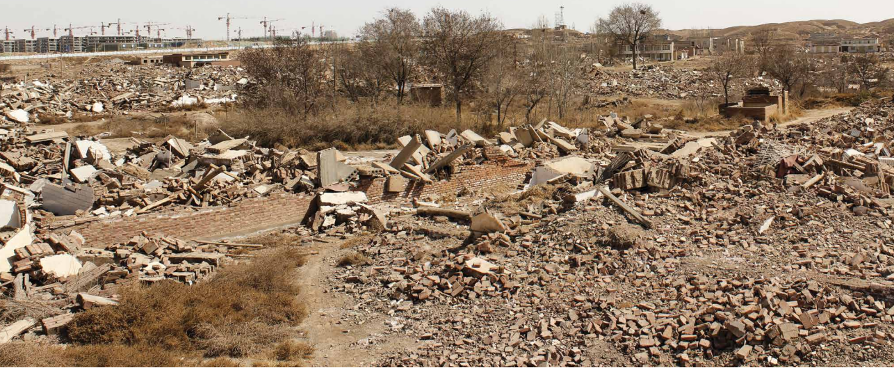
Fig. 5.12: Shanqidun Village in the southeast of the New Area has been completely dismantled and turned into a vast field of debris. In the background on the left are construction sites of new buildings, while on the right, excavators are scraping off hills to create flat ground for development; March 2019.
