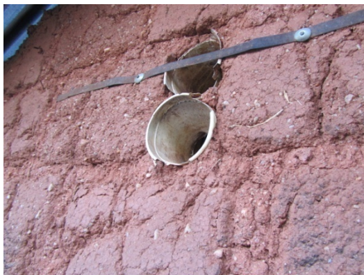
Fig. 6.17 Permanent vents made from the 500gm Kasuku .
