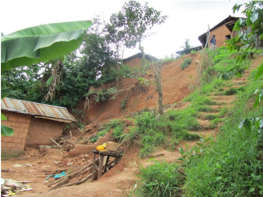
Fig 5.11 House buried by a collapsed embankment. This house a few kilometers from study area of Mihuti resulted in one death in May 2012. (Source: Author, 2012)
