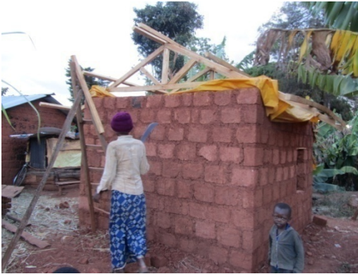
Fig. 6.16 Small room for a kitchen build with mud blocks and trussed waiting for the GCI sheets.
