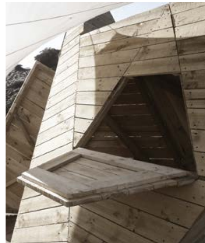
Las Piedras del Cielo. Åpninger inn i kjøkkenrommet. Las Piedras del Cielo. Openings into the kitchen room.
