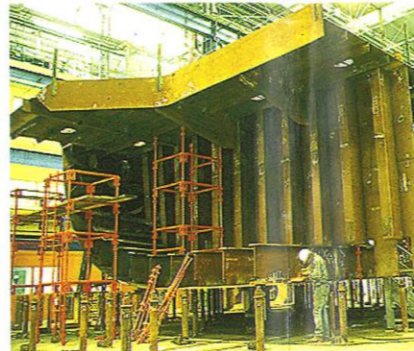
workers weld plates and profiles to sections. Cut edges are milled so that welded plates will fit perfect together.
