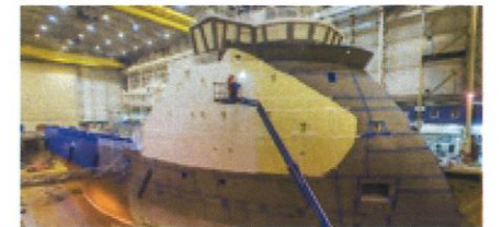
Paintshop. We offer prepaint surface treatment of hulls and hull parts, including sandblasting and waterblasting. The painting process is performed in the controlled indoor environment of our dockhall.
