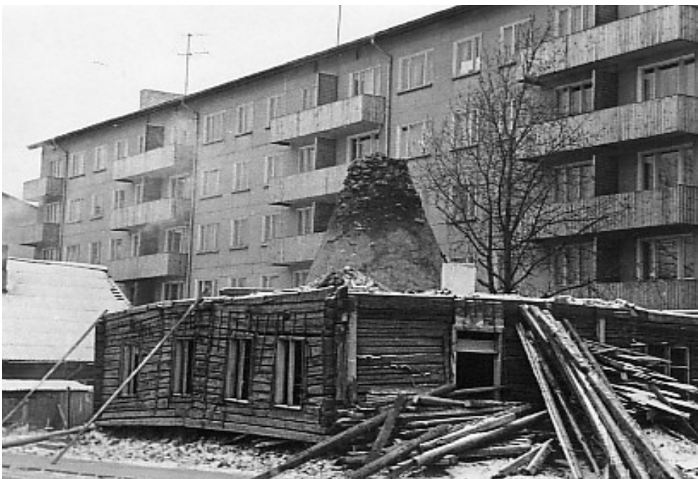
A 18th century vanabalti maja being torn down in front of a newly built Khrushchyovka at Pärnu street 8 in Paide. Many of these early urban dwellings were built close to city centers and were often demolished as to make way for buildings with higher densities.
