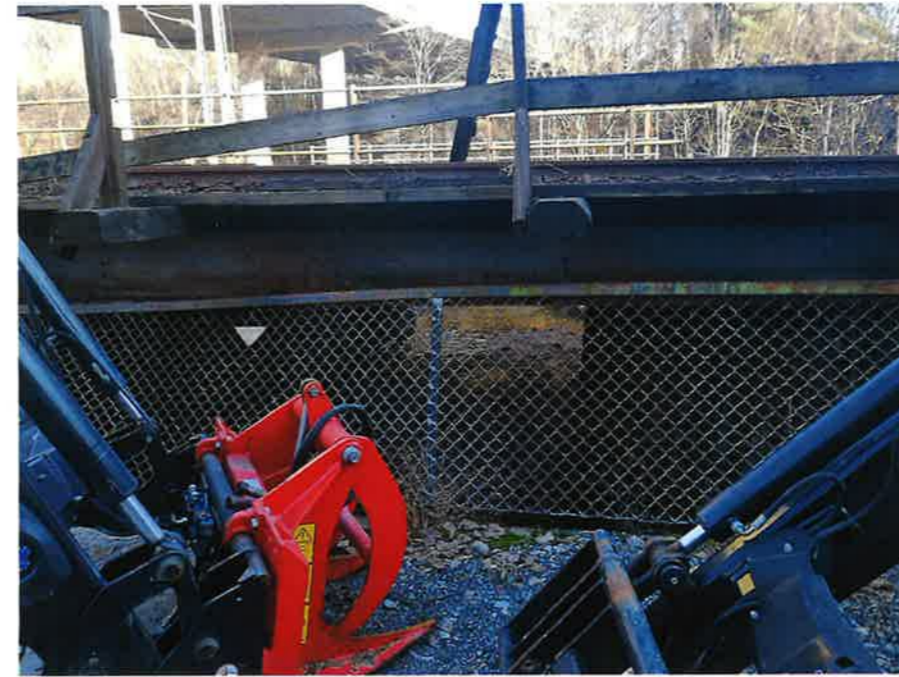
27. The river enters the pipes after running under the bridge for the trams
