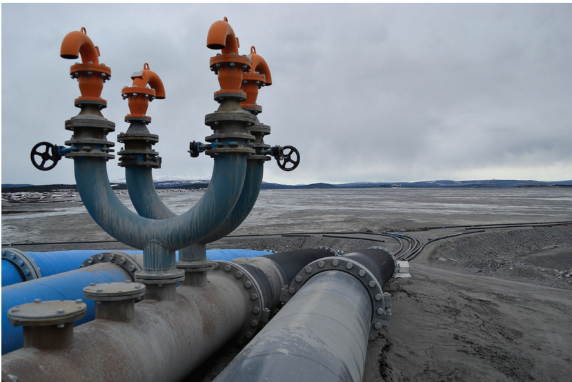
Fig 4.10: The image shows the outlet of the Mine tailings disposal in Aitik. From Naturvernforbundets excursion to the North Calotte.
