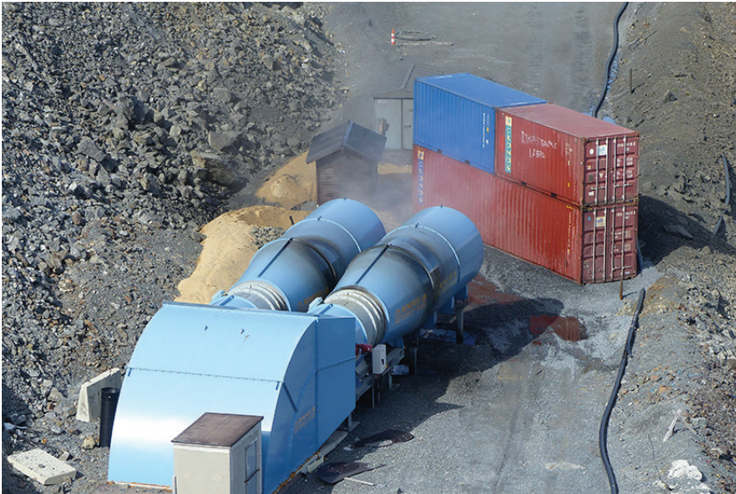
Fig 4.11: Ventilation outlet from the underground gold mine in Kitåla. From Naturvernforbundets excursion to the North Calotte.
