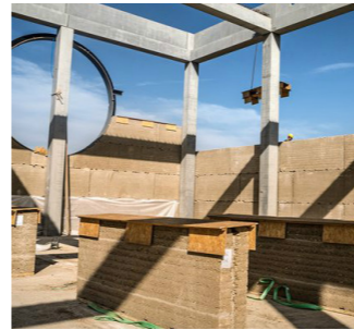
Ricola Krauterzentrum by Herzog & de Meuron, 2014. Rammed earth façade and prefabricated concrete loadbearing structure.
