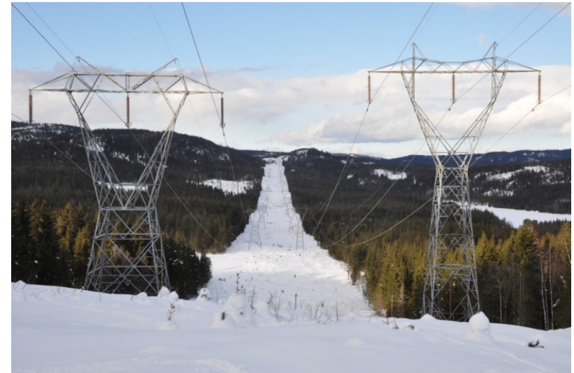
Fig. 38: High-voltage wires cutting through the landscape
