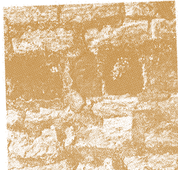
Figure 15.8 Parish church, Bedfordshire, England The poor pointing breaks up, because it is too hard. The cement mortar has been spread too thickly, over the joints but not treated deeply enough - it has accelerated the decay of the stone
