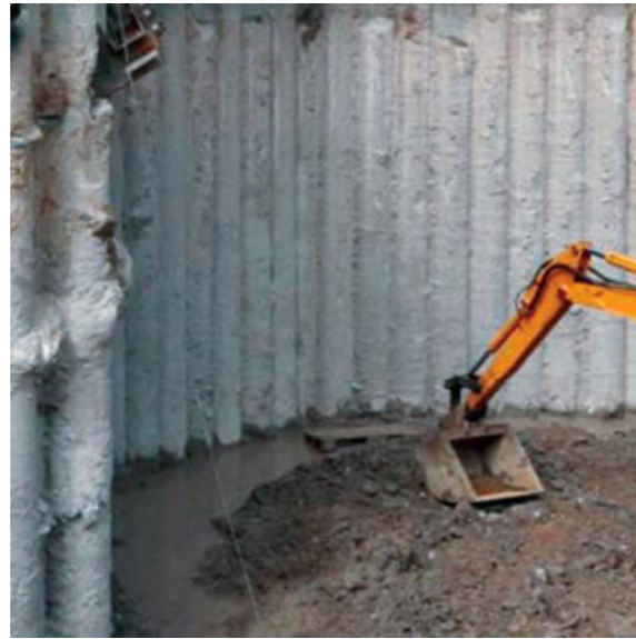
Left: The landscape architecture office BOGL has been using the same technic as secant pilling, a on site concrete casted pill to stabilize the ground seen to the right. The method is call secant pilling. BOGL has by casting the c oncrete in soil form a pattern of concrete islands that creates a new geology.
