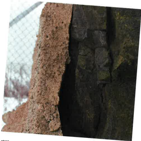
TUNNEL A CONCRETE LAYER IS ADDED TO THE BASALT ROCK MATERIAL - HIDDEN DRIED BEHIND IT - CONTRAST
