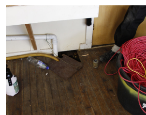
Hole in the floor for cleening
