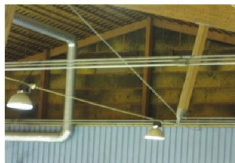
Fig. 2. Mould growth on the ice rink structure.
