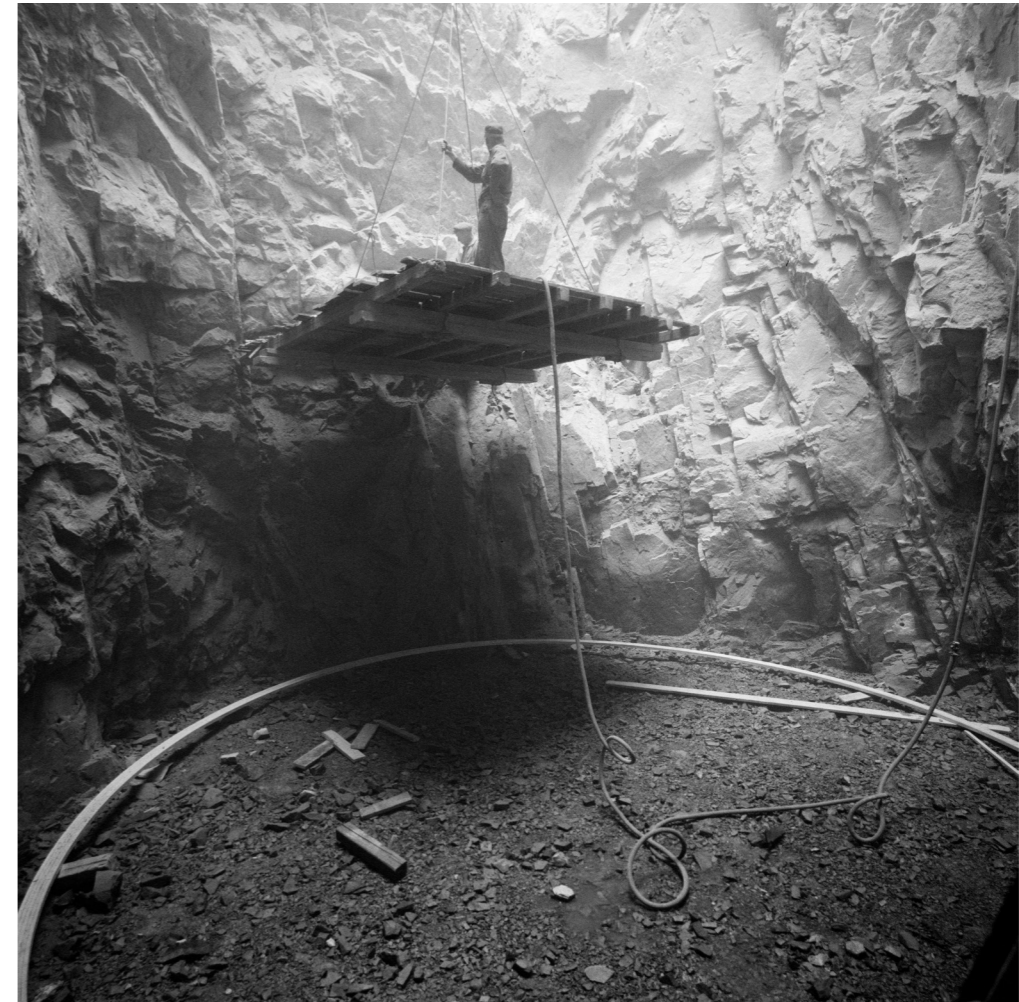
Construction started by digging a 30 meter deep hole for the concrete foundation. Construction, 19.10.1959 Knudsens Fotosenter, Norwegian museum of science and technology
