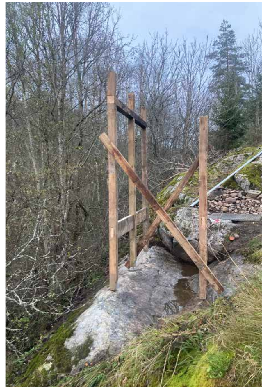
The beams are embedded into the columns and secured with a dowel.
