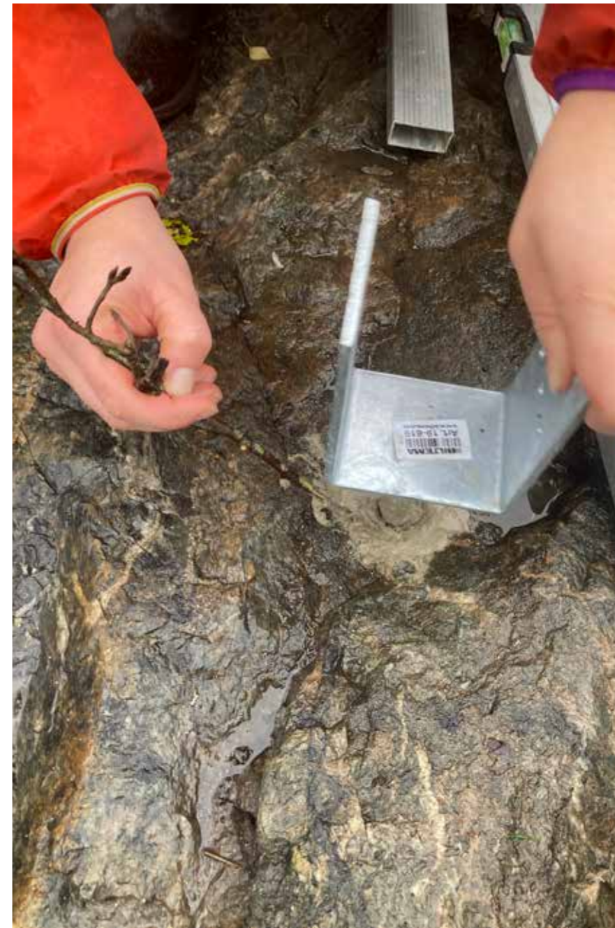
A star-shaped hole is the result of drilling in an existing hole. Pouring the concrete before placing the pin was the wrong order of doing things.
