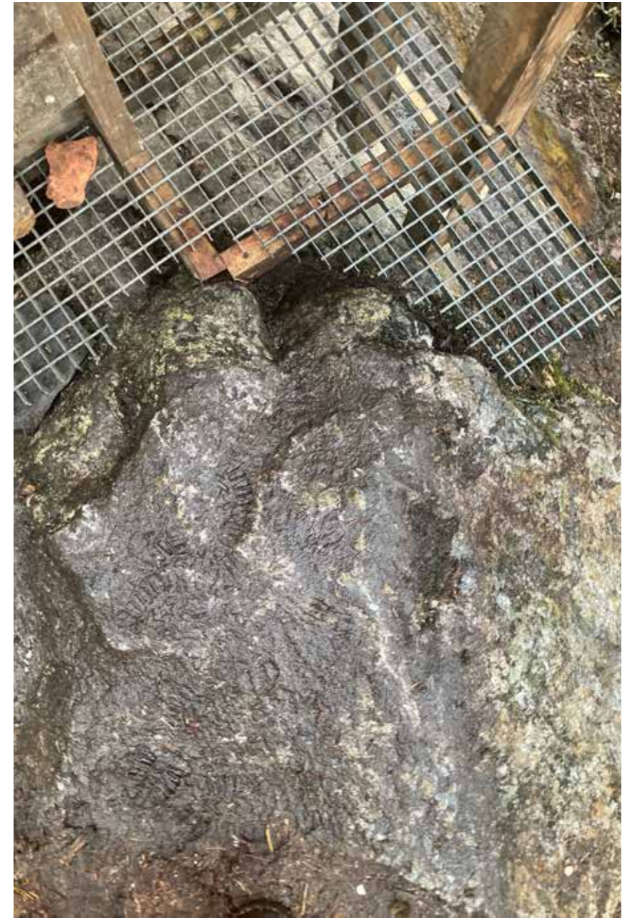
We added stone from clearing the site to level the entrance area where the elephant grate extends out of the building and hits the bedrock.
