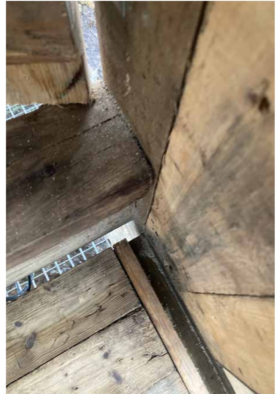
Tracks for planned screens to be pushed back and forth on wheels. To regulate visibility and sun.
