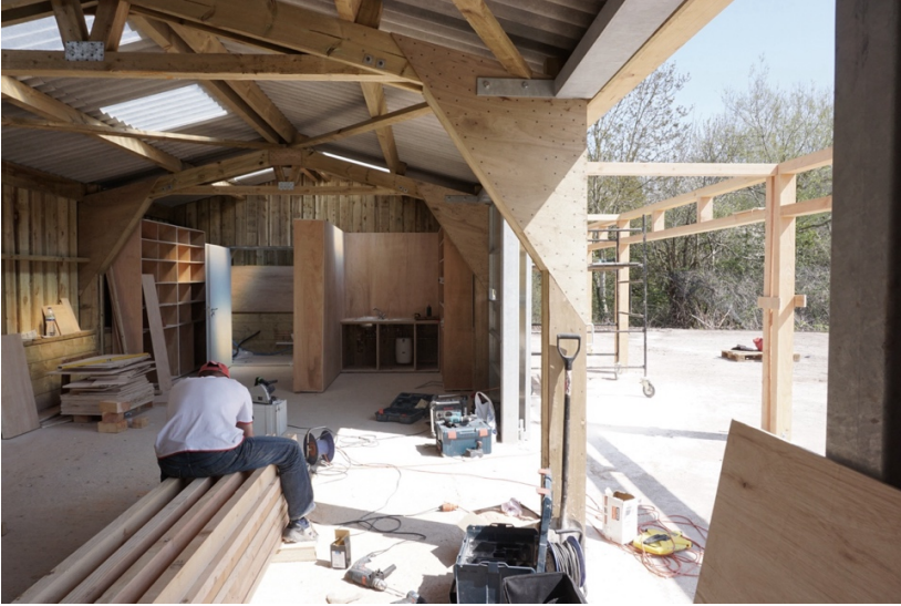
Figure 4. Building Site, Avon Wildlife Trust Cabin, Bristol, Hugh Strange Architects. 2015. (Photo: Hugh Strange)
