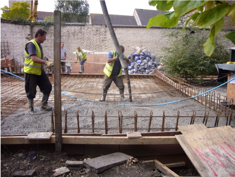
Figure 4. Concrete slab poured on top of existing slab by the main contractor. Strange House, London, Hugh Strange Architects. 2010. (Photo: Hugh Strange)
