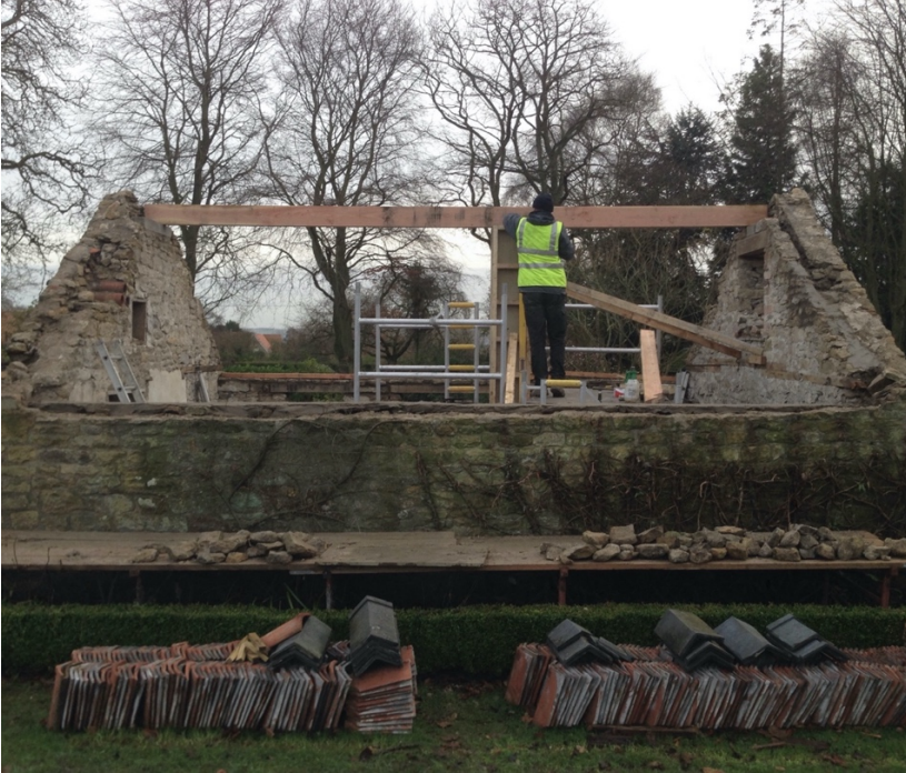
Figure 5. Building Site, Harewood Studio, North Yorkshire, Hugh Strange Architects. 2016. (Photo: Hugh Strange)
