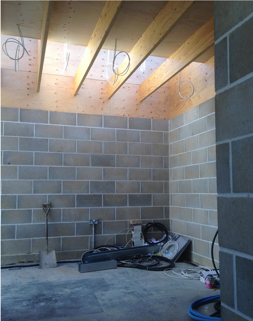
Figure 7. Building Site, Garden Room, London, Hugh Strange Architects. Completed 2019. (Photo: Hugh Strange)
