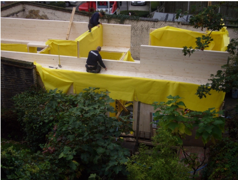
Figure 2. CLT, fabricated in a factory in Switzerland, erected on site in 48 hours. Strange House, London, Hugh Strange Architects. 2010. (Photo: Hugh Strange)
