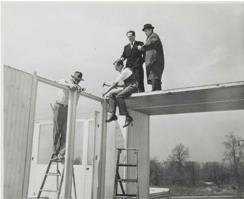
Figure 11. Walter Gropius and Konrad Wachsmann on site with the prototype Factory-made House
